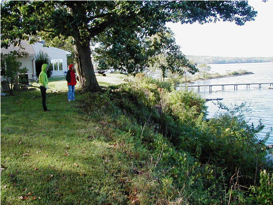
Historical photograph taken facing south showing a failing slope that was slumping; October 10, 2010.
