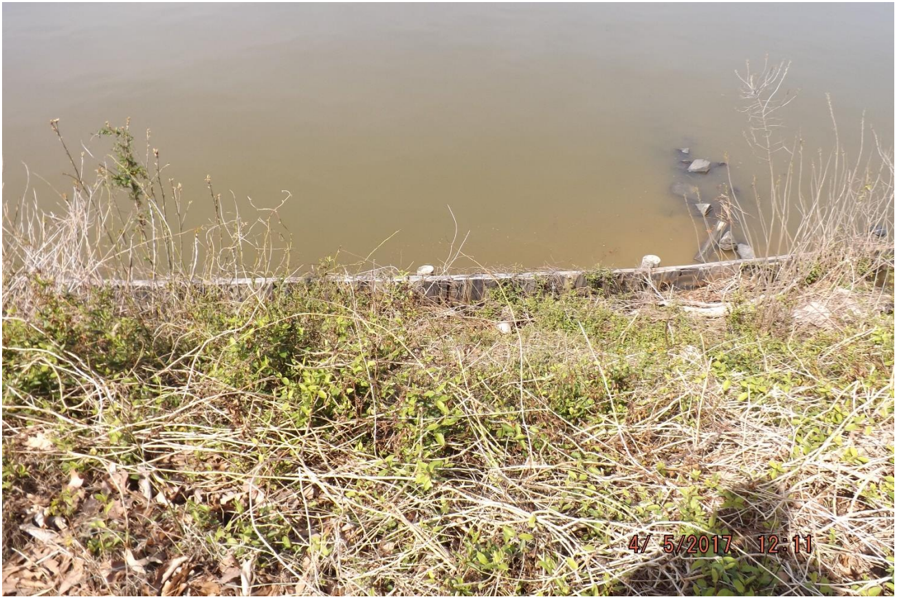
Historical photograph taken facing west showing a failing slope that was slumping and a failing bulkhead; April 5, 2017.
