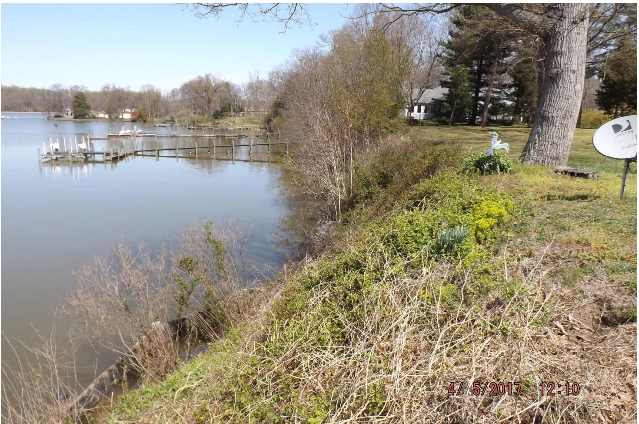
Historical photograph taken facing north showing a failing slope that was slumping and a failing bulkhead; April 5, 2017.
